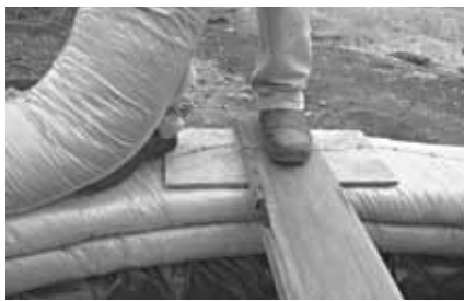
Above: Cantilevered stair treads were inserted between rows to a depth of 300mm. Right: Forms were built using scrap wood.
